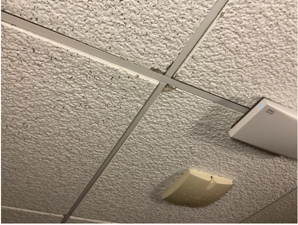
Acoustical tile deterioration
