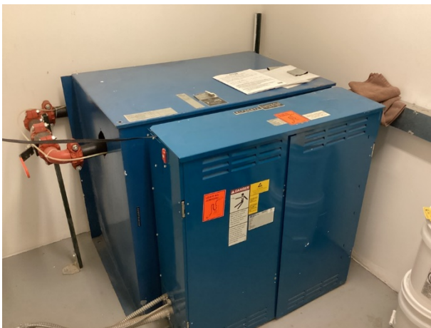
Hydraulic elevator equipment
