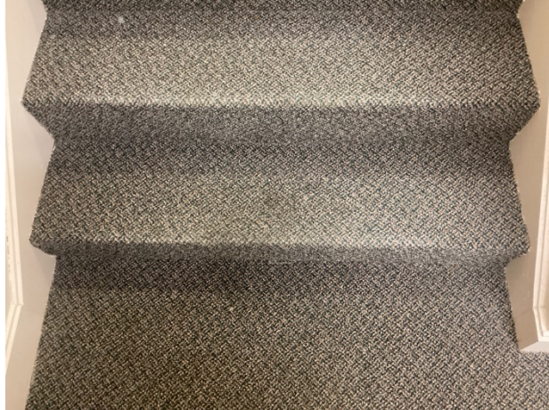
Stairwell carpet deterioration
