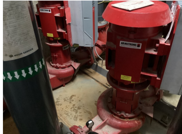
Cooling tower pumps
