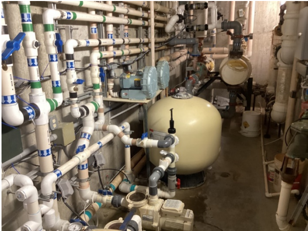
Pool mechanical equipment
