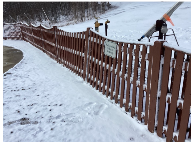
Fence leaning section
