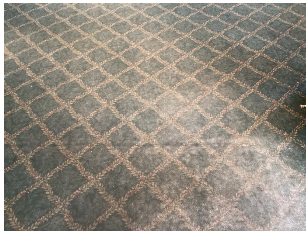
Lobby carpet deterioration
