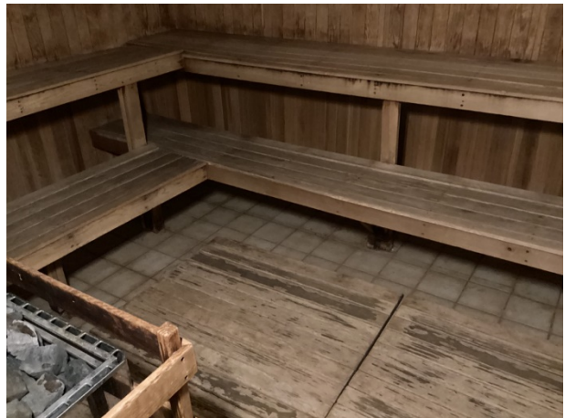
Sauna finishes Note: General wood deterioration.
