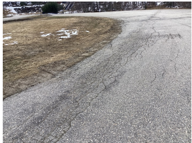
Edge deterioration and alligator cracks at upper parking area
