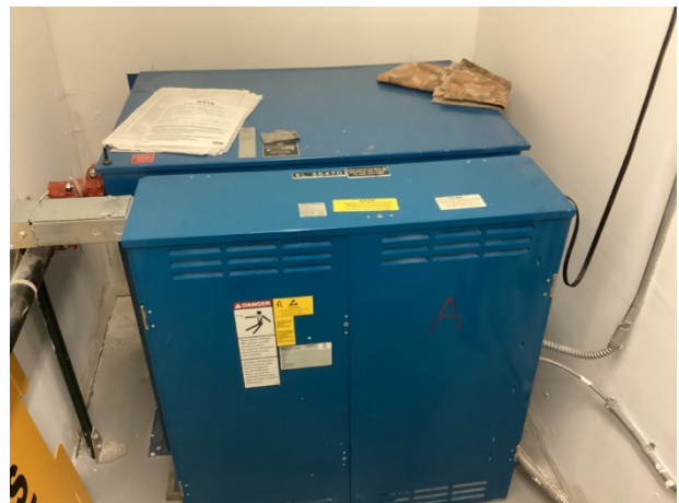
Hydraulic elevator equipment
