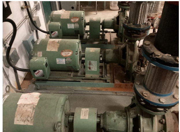
Building cooling pumps
