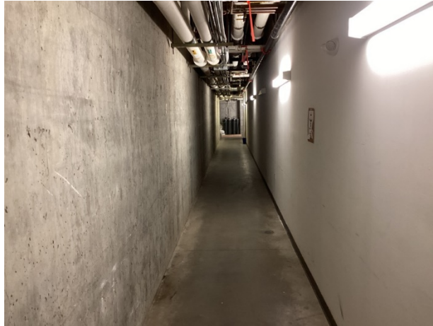
Service corridor overview
