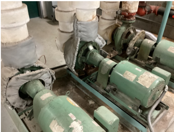
Building heating pumps
