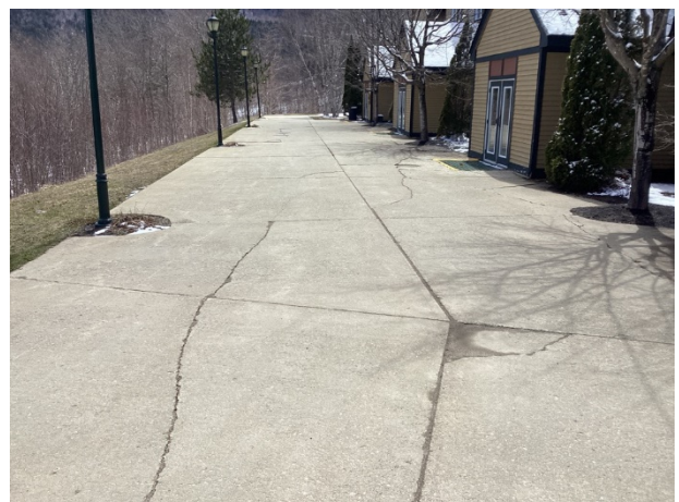
Sidewalk overview with cracks and settlement
