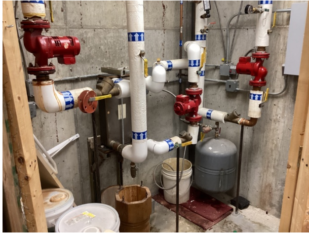
Deck heat exchange system
