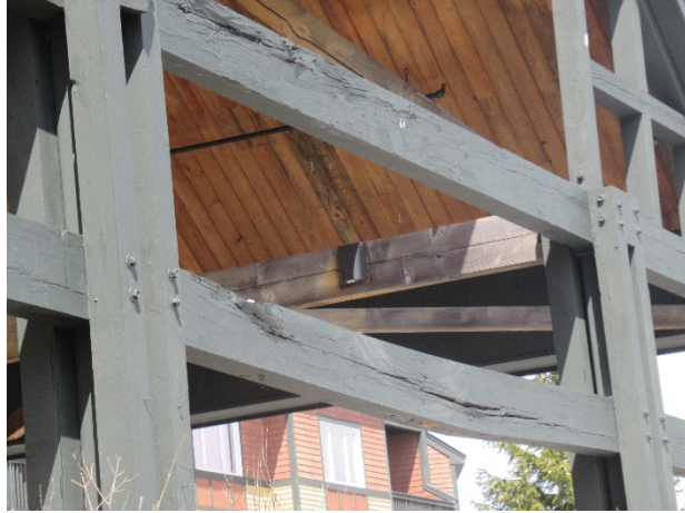
Wood split and rot and portico beams
