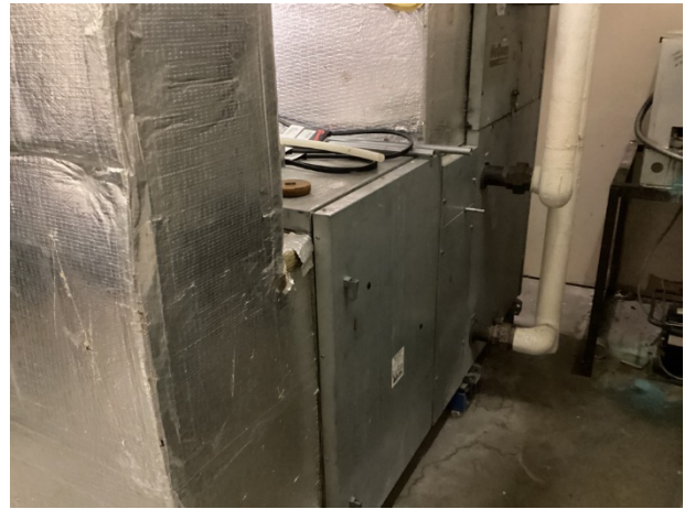
Make-up air unit
