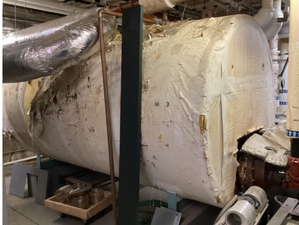
Common storage tank
