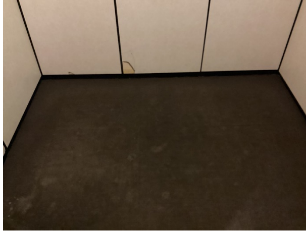
Elevator cab finishes Note: Carpet stains and wall damage.
