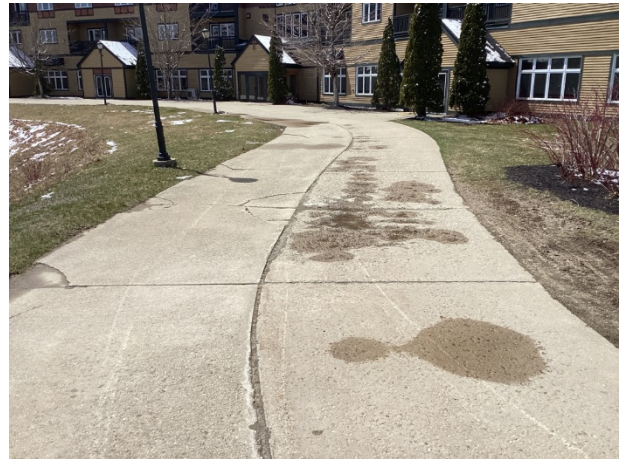
Sidewalk overview with cracks and spalls
