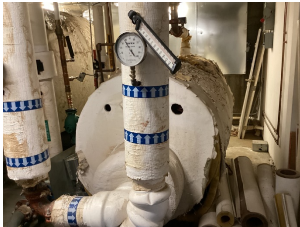
Shooters storage tank
