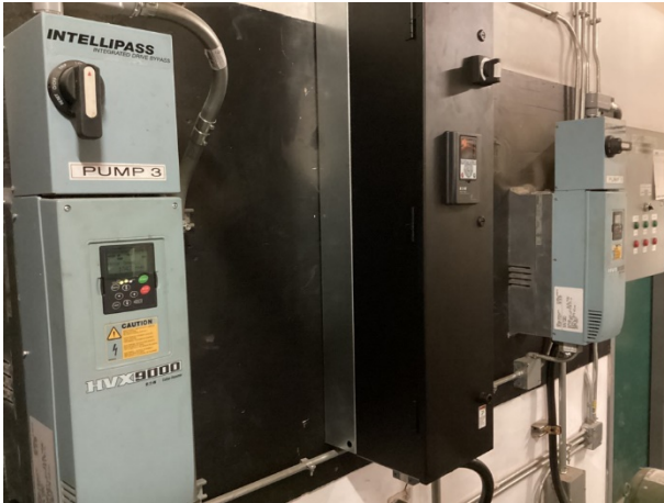
Cooling pump VFDs
