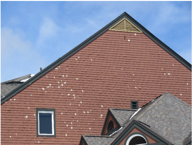
Siding overview with finish deterioration and displaced shakes
