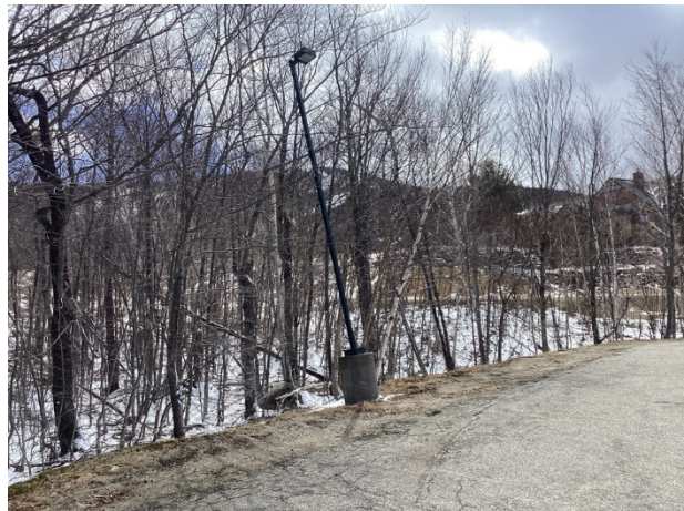
Leaning light pole and fixture
