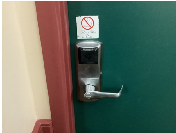
Guest room access control system
