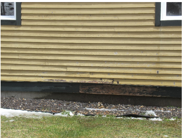
Siding rot and finish deterioration
