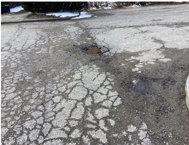
Alligator cracks at upper parking area
