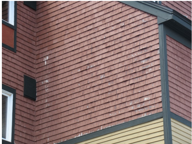
Siding finish deterioration and warp
