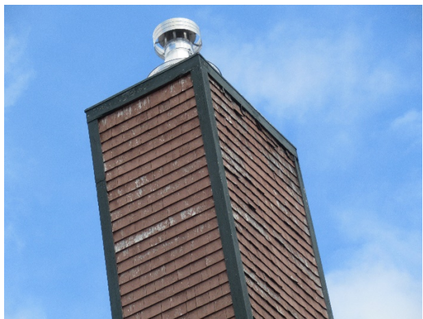
Siding deterioration and finish deterioration at chimney chase
