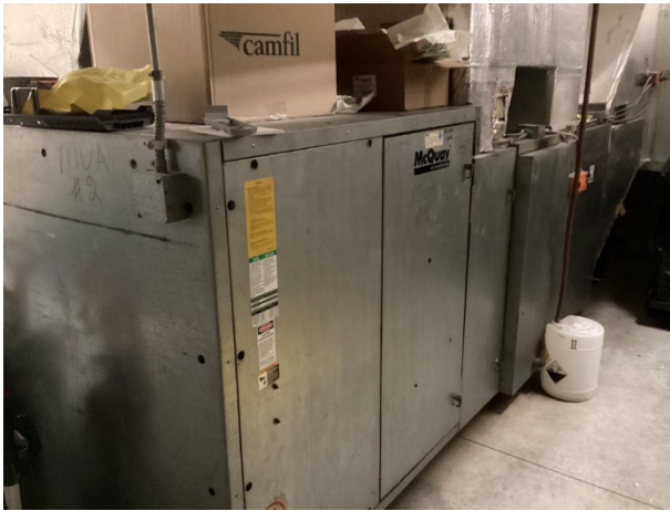
Make-up air unit
